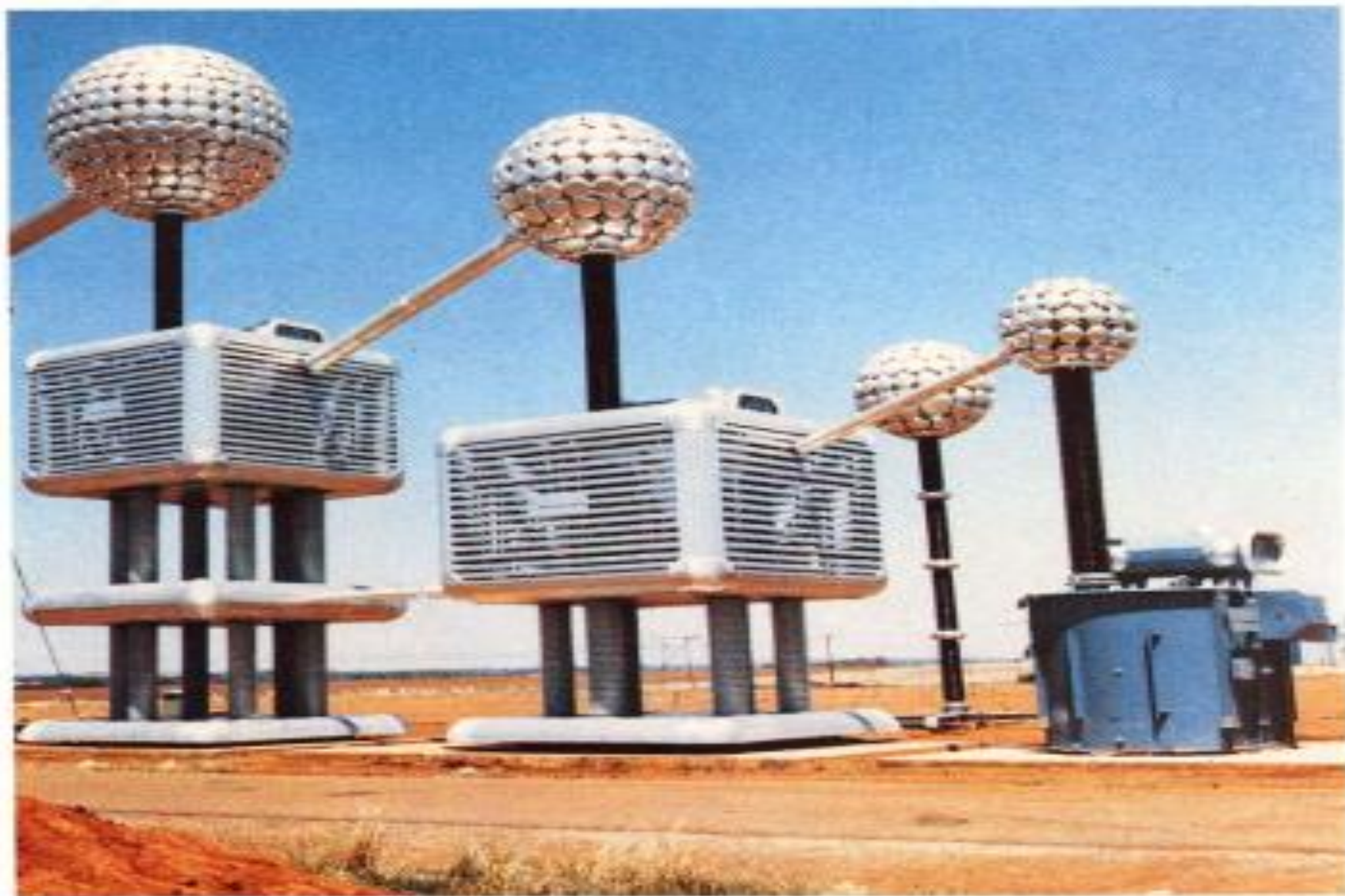
Three-stage cascade transformer 3 x 600 kV, 2 A cont. outdoor type with AC voltage divider 1500 kV
